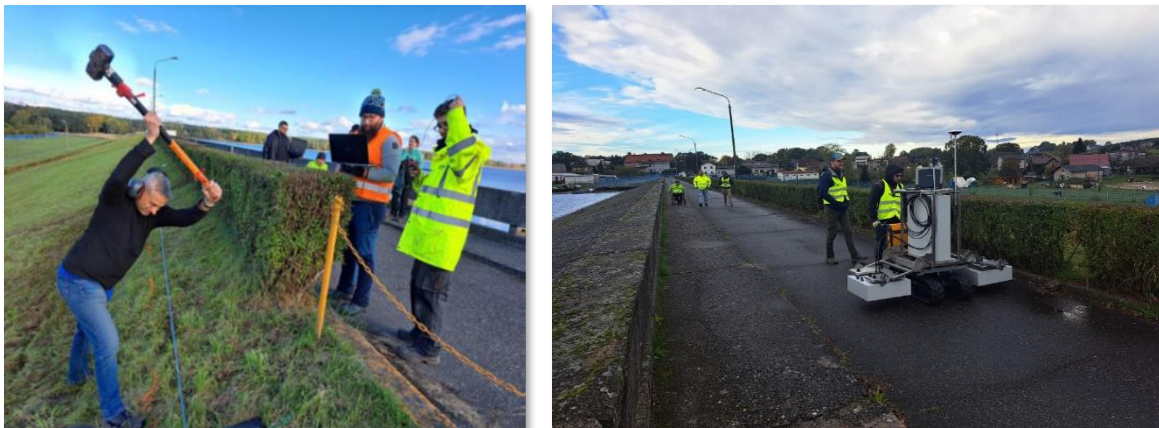
Fig.2 A combination of near-surface geophysical methods (seismic tomography and imaging, GPR, ERT) were used to image the structure of the dam. Seismic survey based on standard geophones supported with additional fiber optic sensor (DAS). All measurements were planned as time-lapse survey to catch temporal changes. Seismic measurement with sledgehammer source (left), spectral georadar (right).
